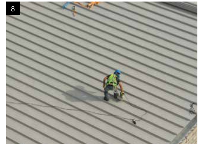
8. Standing seam sheets are installed on the halters and zipped by a zipping machine.
