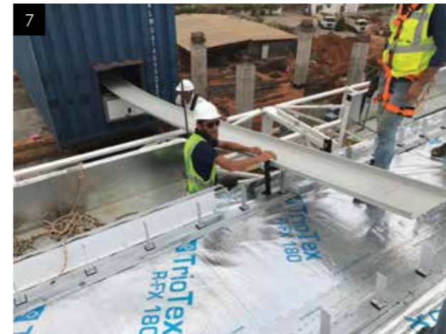
7. The 75m long standing seam sheets produced on roof level. The rollformer lifted on the eave level by a special scaffolding.
