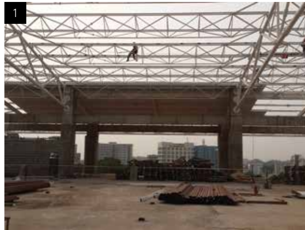
1. Before commencing the execution of decking, Lambda checks the steel structure by surveyor if it is within the tolerances or not. Safety comes first according to Lambda site execution policy, therefore fall protection safety system is set before starting the installation.
