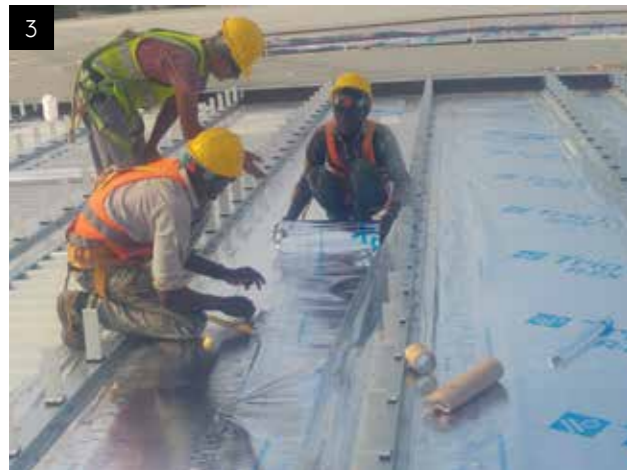
3. Vapor control layer is installed in pieces together with the top hats to prevent the tearing risk during the installation of halter clips.
