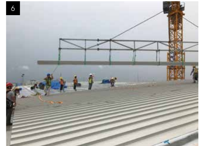
6. The standing seam sheets up to 44m is produced on ground level and lifted to roof by crane and lifting beam.
