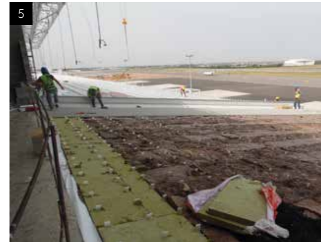
5. Installation of insulation starts whenever vapor barrier, top hats and halters are completed. Around skylights and gutters rigid insulation is used whereas in the middle soft compressable insulation is used.
