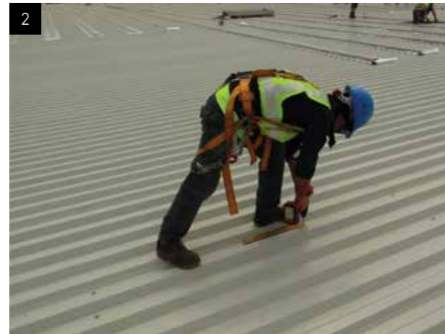
2. The roof decks are installed on purlins by stainless steel 12H-5,5X40 screws.
